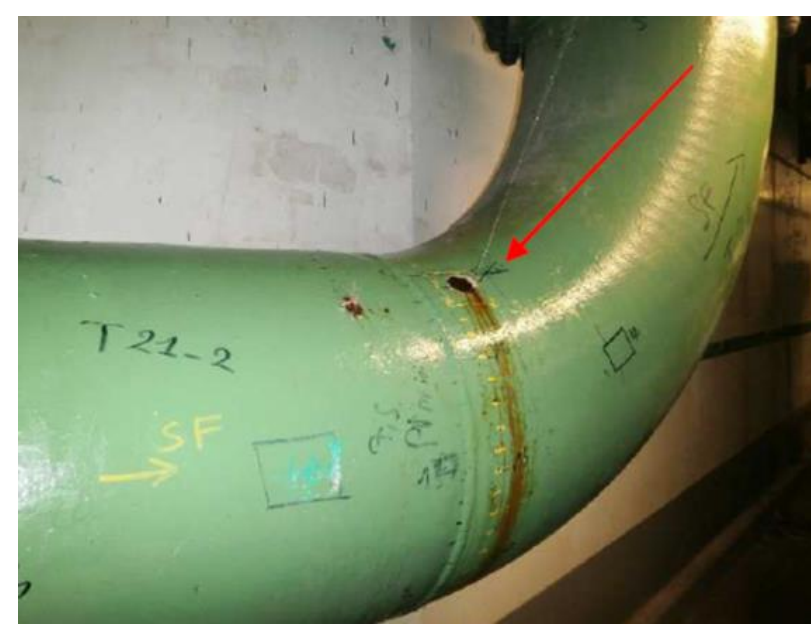
Raw feedwater line of Gravelines plant with leak due to crevice corrosion
