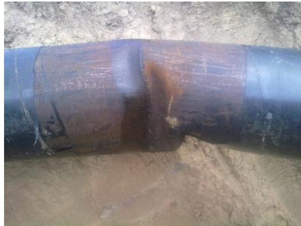
Oil & gas transport pipe
